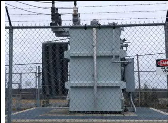
10 MVA Substation Transformer
