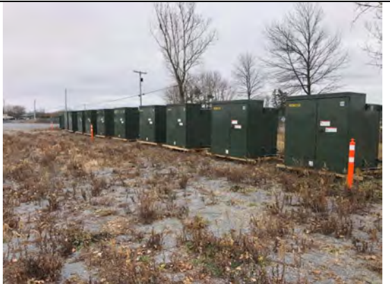
Replacement 208-V/34.5-kV/1-MVA WEG transformers
